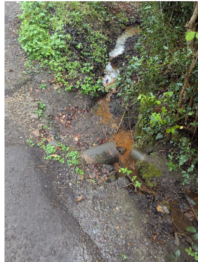
Drainage ditch at north east corner of the central land parcel. Water pipe beneath the Roundabouts Farm access track
