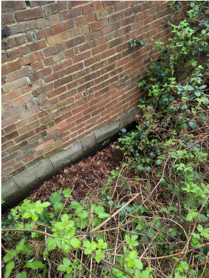
Copthorne Common Ditch at the south west of the northern land parcel
