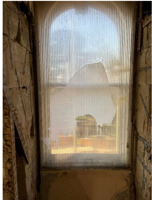
Type 2 - W2.01 with loss of glazing and polycarbonate sheeting both sides
