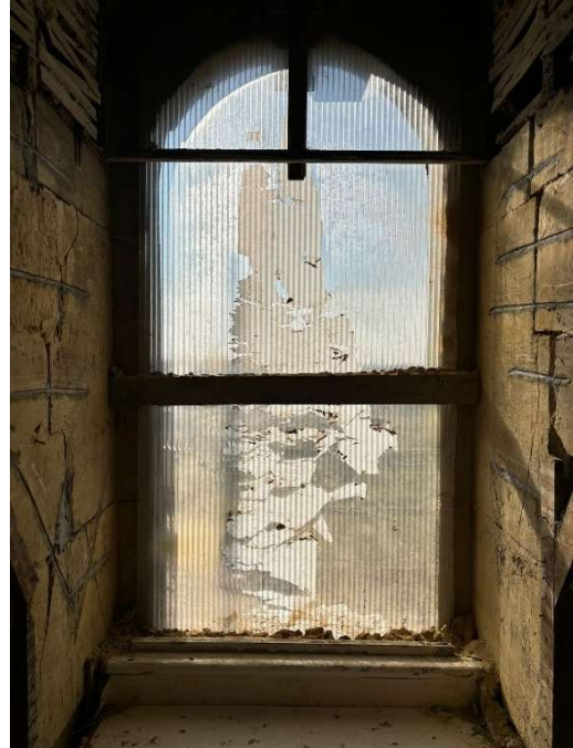
Type 2 – W2.06 with missing frame etc
