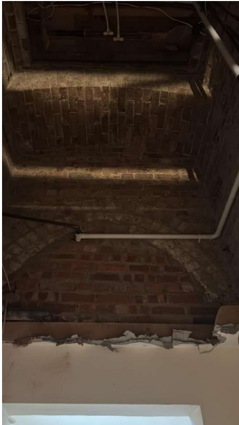
Modern plasterboard ceiling with new pipework run in void above.
