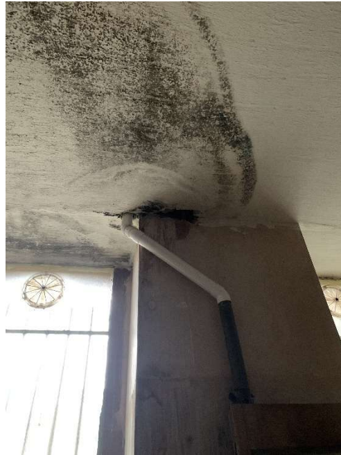
Modern, harmful pipework addition
