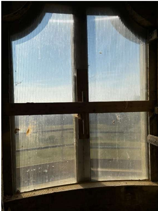
Type 1 – W2.04 with missing frame / glass
