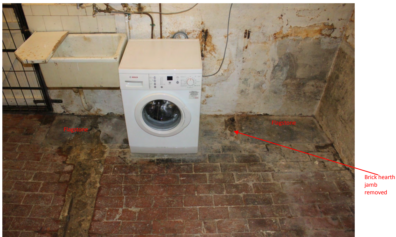
Plate 39. Scars of a missing fireplace and chimney stack.
