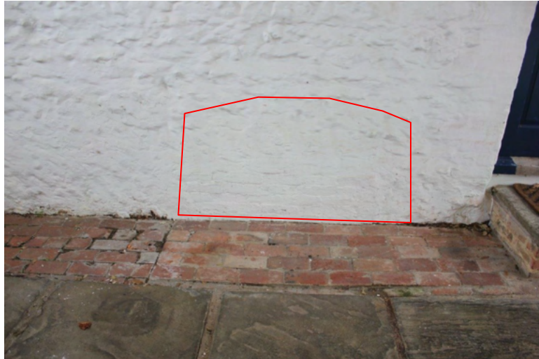
Plate 9. Blocked coal chute aperture in the south elevation.
