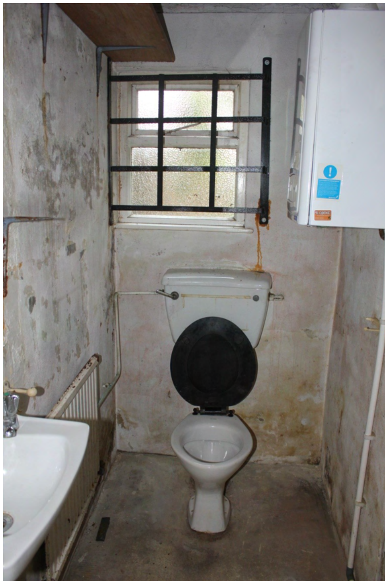
Plate 43. 20 th century sanitary ware and inserted window.
