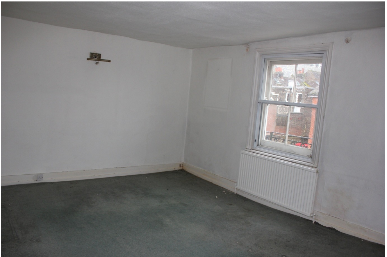
Plate 51. Bow in the floor of Room F4.
