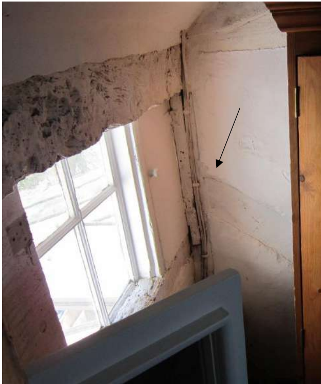
Figure 10; a down brace on the cross-frame between bays 2 and 3
