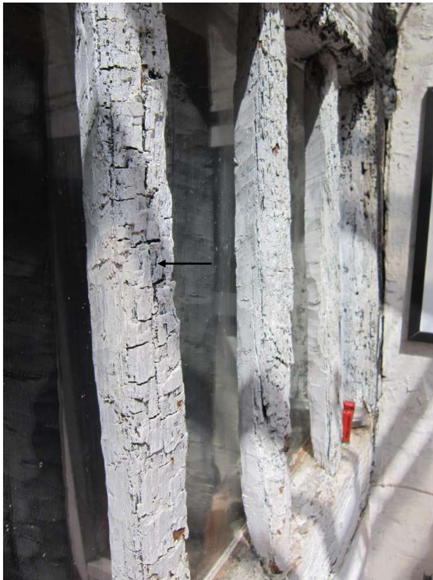
Figure 38; Cuboidal cracking on an external face of a hall window mullion.
