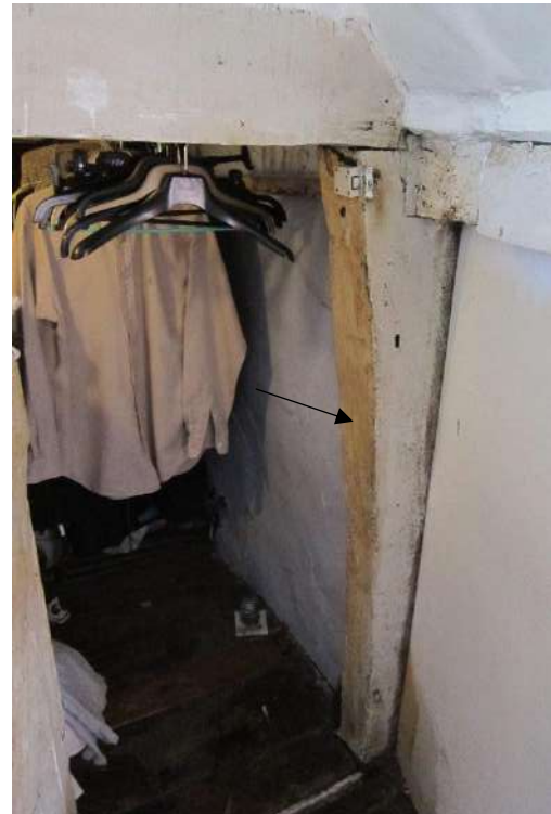
Figure 11; no evidence for a down brace on the cross-frame between bays 1 and 2.
