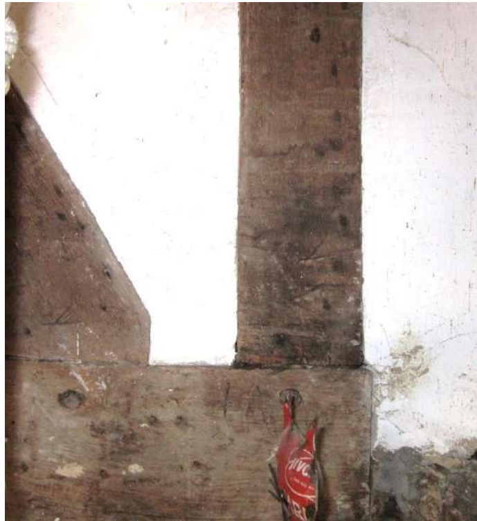
Figure 21; detail of a down brace, stud and girt on this cross-frame between the smoke bay and the lean-to, showing a lack of weathering and visible carpenter's assembly marks.
