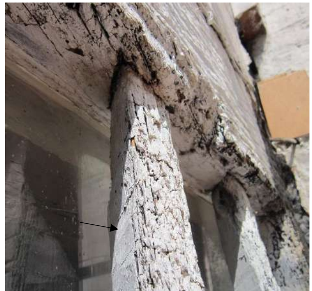
Figure 19; showing a roughly hacked surface of a mullion.
