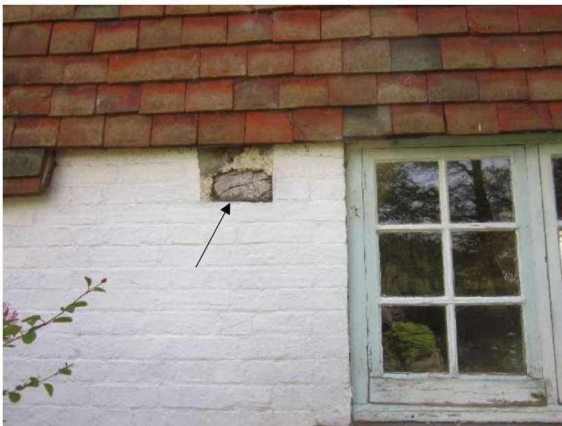
Figure 28; western end of the Phase B mantlebeam almost protruding to the external face of the underbuilt in brick, west wall.
