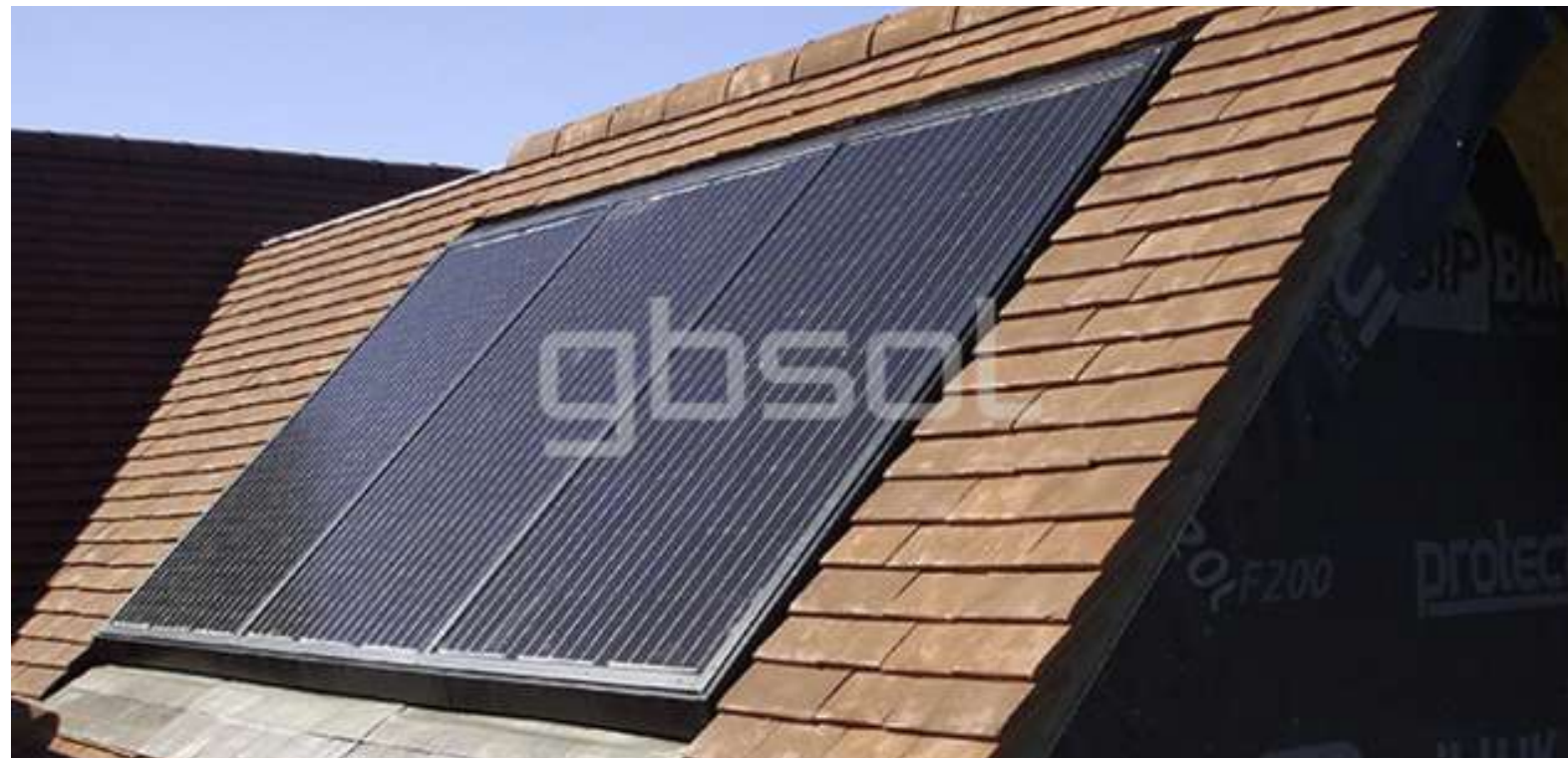
Integral PV's flush to roof
