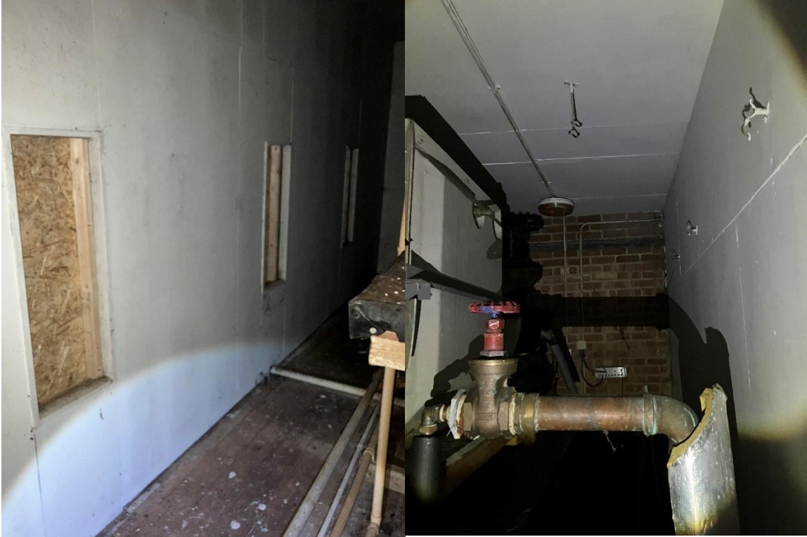
Photo 5: Internals 072 Tank Room
