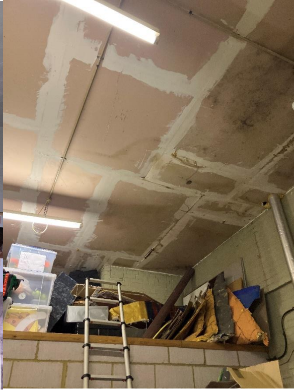
Photo 8: Internals 074 access room
