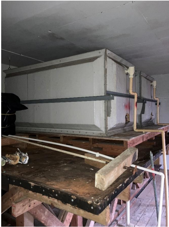
Photo 7: Internals 072 Tank Room (redundant water tanks)
