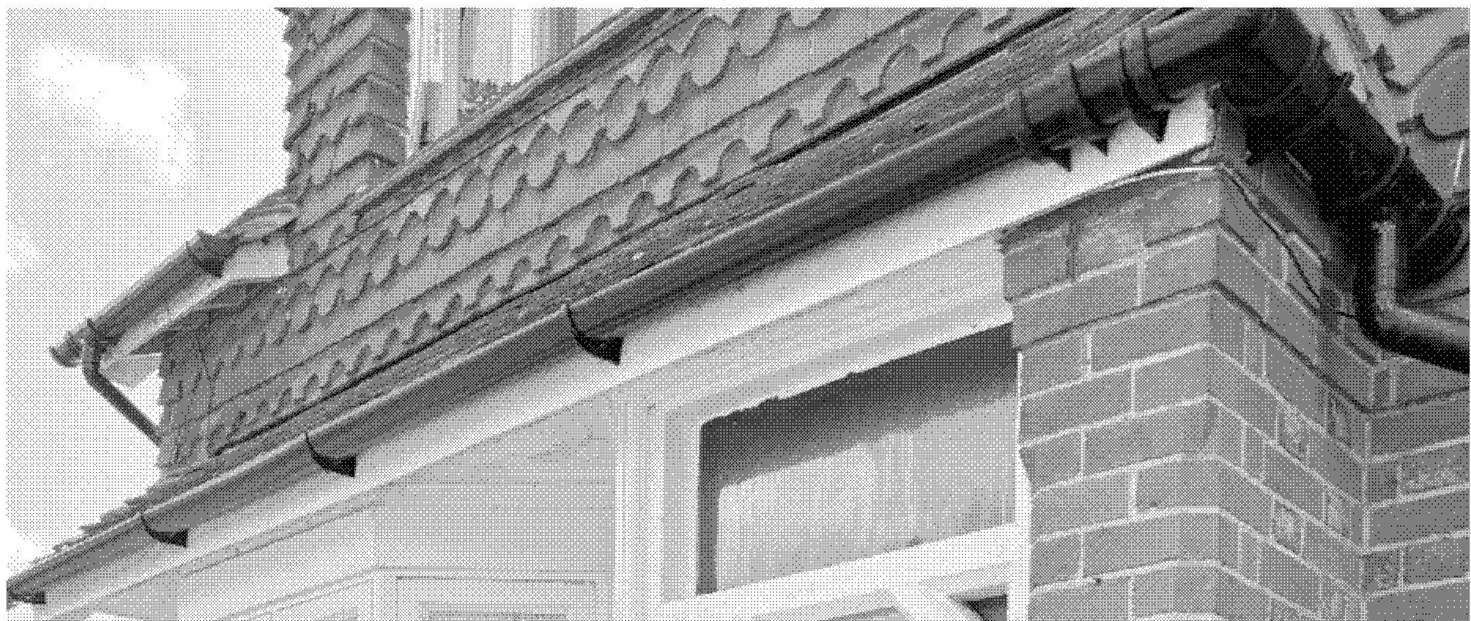
Fig 8: Existing black plastic gutters and downpipes.
