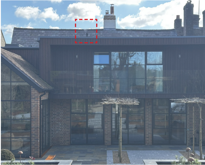
Recent photograph capturing the new boiler flue
