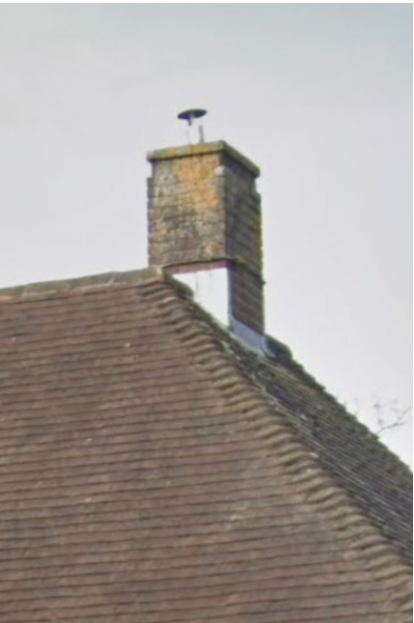
Chimney at Mulberries shows a lack of traditional details: poor flashing installation, no chimney pots and unsightly lichen growth.
