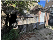
PHOTOGRAPH OF DILAPIDATED TIMBER-CLAD OUTBUILDING
