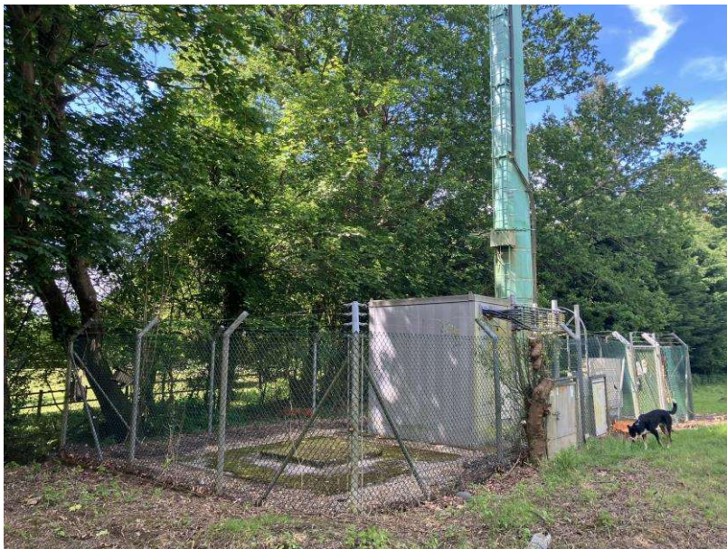
Photo of existing telephone mast and infrastructure.
