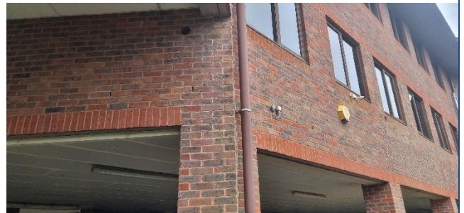
Photo 4: North Eastern Corner of the Building, Showing Consistent Weep Hole Features and Open Air Vents.
