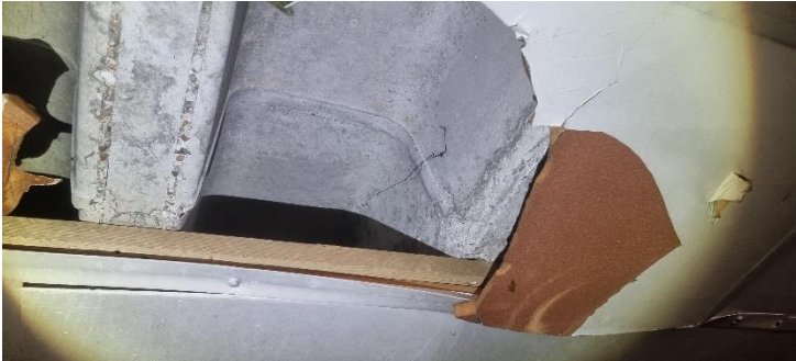
Photo 5: Gaps Present in the Ceiling of the Undercover Carpark Area to the North West of the Building.
