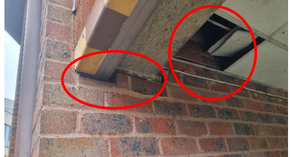
Photo 2: PRFs Present within the Ramped Carpark Area
