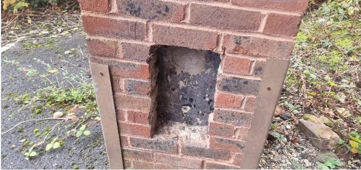
Photo 1: Brickwork Inspected with an Endoscope on the Northeastern Corner of the Building.
