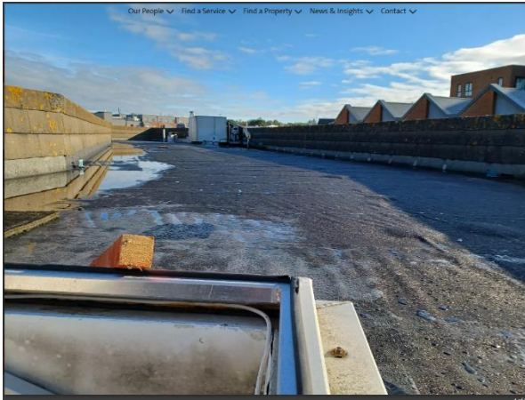
Photo 20: Image from the Flat Roof
