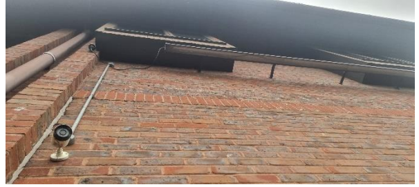
Photo 17: Gap Present Underneath the Window on the Southeastern Elevation of the Building.
