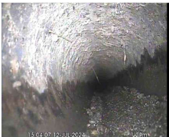
MANHOLEX_eaa616f7-975f-4e97-ac3b-557e21e09b41_20240725_102200_152.jpg, 00:00:38, 1.29 m Settled deposits, fine, 10% cross-sectional area loss
