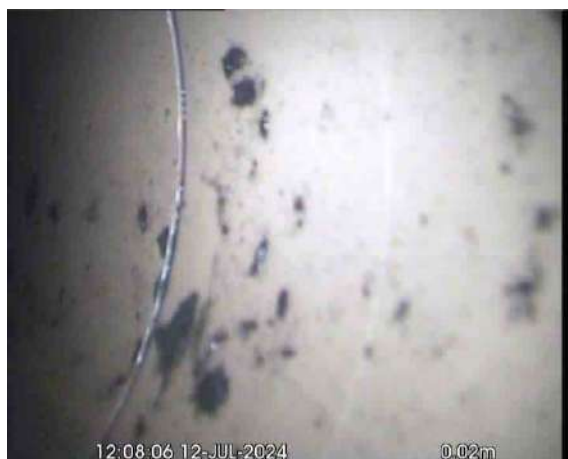
CAPPED OFFX_2c61c11e-4c06-4ebc-870a-c78b293b4c99_20240725_093434_293.jpg, 00:00:43, 0.02 m Line deviates left
