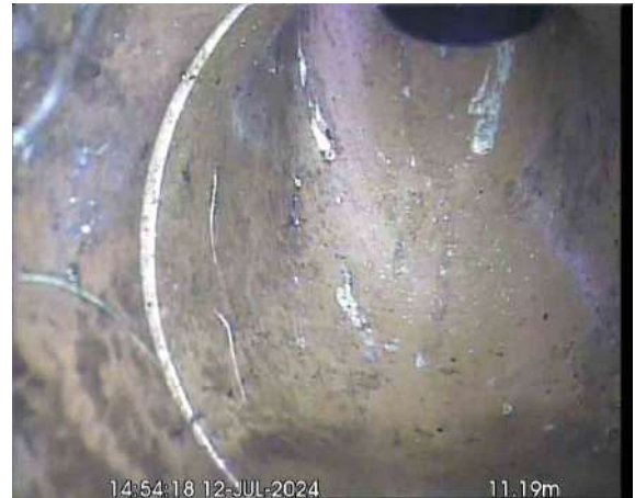
RWDPX_86dc6ebb-da85-45a0-a40c-1b8118d31bb7_20240725_101744_768.jpg, 00:01:49, 11.19 m Line deviates up, REST BEND
