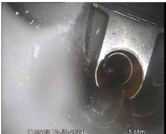
MH2X_b55e55f8-9e05-4db8-b212-fbb573044cff_20240725_093147_156.jpg, 00:01:29, 5.68 m General remark, **ENTERS MANHOLE 3 (MH3) - UNABLE TO LIFT
