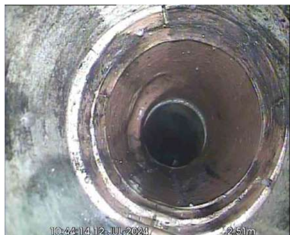
MH6X_5b7b7237-2ba3-4cba-86aa-fcb1f22d1ecc_20240725_092232_813.jpg, 00:00:41, 2.51 m Fracture, multiple at joint from 12 o'clock to 12 o'clock
