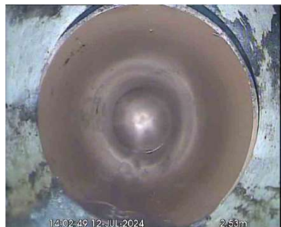
GULLYX_a0d2ed5e-7b7e-4ae5-a077-94c7952a4929_20240725_101329_585.jpg, 00:01:00, 2.53 m Joint displaced, medium
