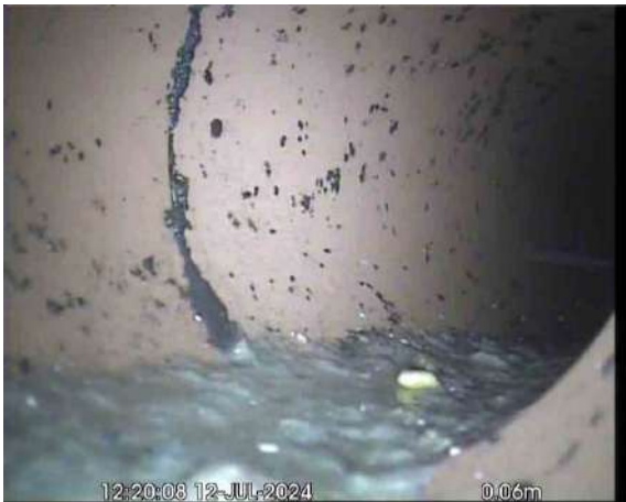
CAPPED OFFX_962b07f7-60c1-43c4-ba8a-1193030da8e6_20240725_094225_233.jpg, 00:00:42, 0.06 m Settled deposits, fine, 5% cross-sectional area loss
