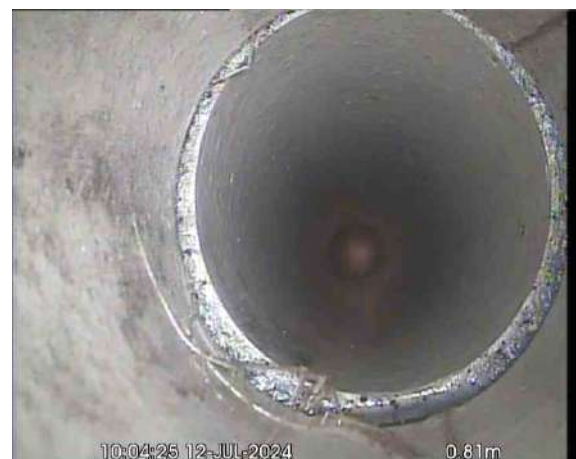
GULLYX_497c7feb-53ee-44b1-89dc-872bd2b7a9cf_20240725_090218_006.jpg, 00:01:01, 0.81 m Roots, fine at joint
