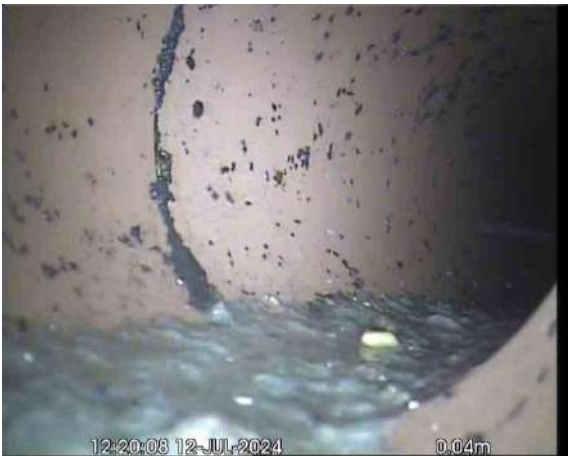
CAPPED OFFX_80832dd5-8ef6-4f5d-89c0-115ac1b2d810_20240725_094214_228.jpg, 00:00:41, 0.04 m Line deviates right
