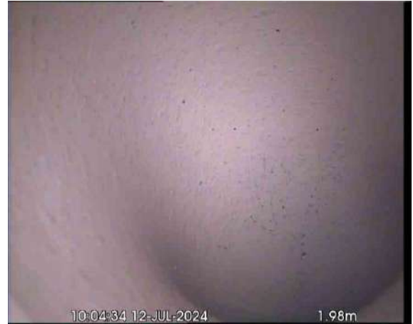
GULLYX_ea8e3b67-ae80-4672-8aa1-6d7696ac026d_20240725_090241_494.jpg, 00:01:10, 1.98 m Finish node, gully, reference: GULLY
