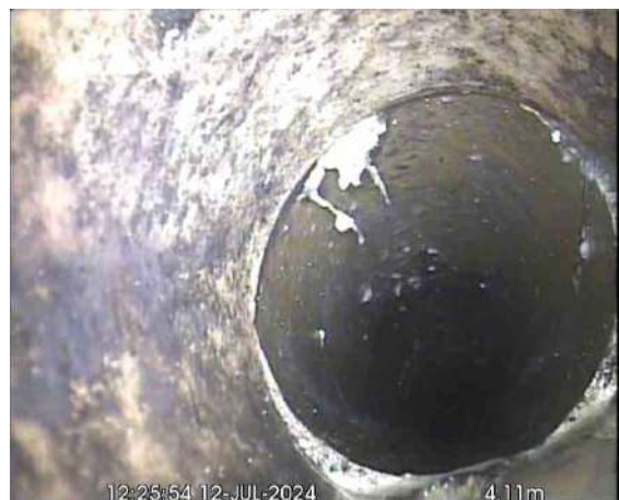
MH5X_059f6707-2778-4d9f-998a-3e91e87c5d40_20240725_094727_709.jpg, 00:01:24, 4.11 m Joint displaced, medium
