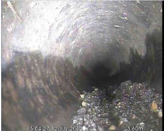
MANHOLEX_3776ed84-49e6-4422-b862-3e0982192f67_2024 0725_102228_650.jpg, 00:00:58, 3.60 m Settled deposits, fine, 10% cross-sectional area loss
