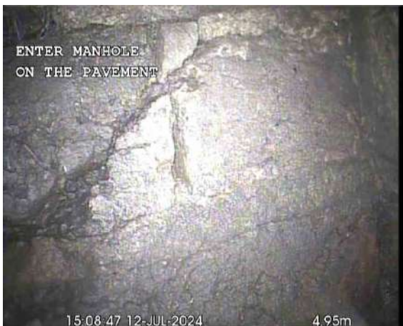
MANHOLEX_fcf897e3-6b5d-4475-8745-3d5110d5f99c_20240 725_102321_800.jpg, 00:01:32, 4.95 m Finish node, manhole, reference: ENTERS MANHOLE ON THE PAVEMENT AREA
