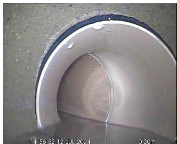
MH2X_9e3848a9-2aef-4403-9dc0-06a55e9cccf0_20240725_092609_653.jpg, 00:00:56, 0.30 m Joint displaced, medium
