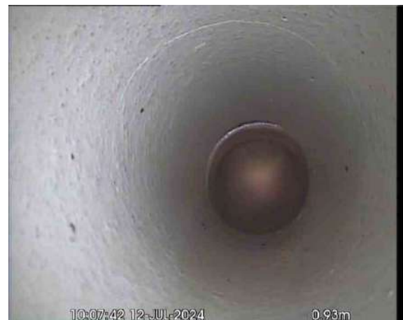
W_CX_9fa16cc0-0598-4ab2-b04a-1bd0e0447c7d_20240725_090647_708.jpg, 00:00:34, 0.93 m Crack, circumferential from 9 o'clock to 3 o'clock
