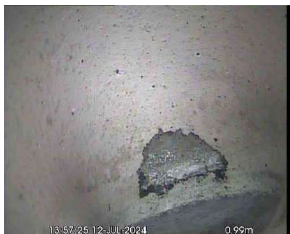
GULLYX_6d63e6bc-a192-46ee-bb28-5b54a1a3e0d8_20240725_095748_794.jpg, 00:00:39, 0.99 m Finish node, gully, reference: GULLY
