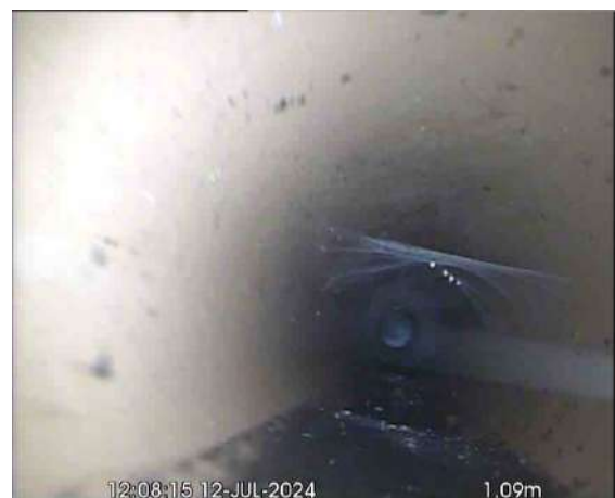
CAPPED OFFX_67eeaf64-0435-43b5-8da3-b5a094747b11_20240725_093450_860.jpg, 00:00:52, 1.09 m Water level, 5% of the vertical dimension
