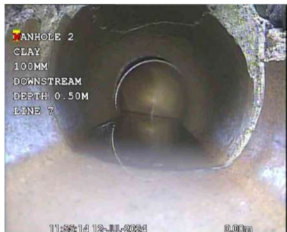
MH2X_71184cee-8274-417a-b5b5-87d394df23a5_20240725_092449_717.jpg, 00:00:28, 0.00 m Water level, 10% of the vertical dimension
