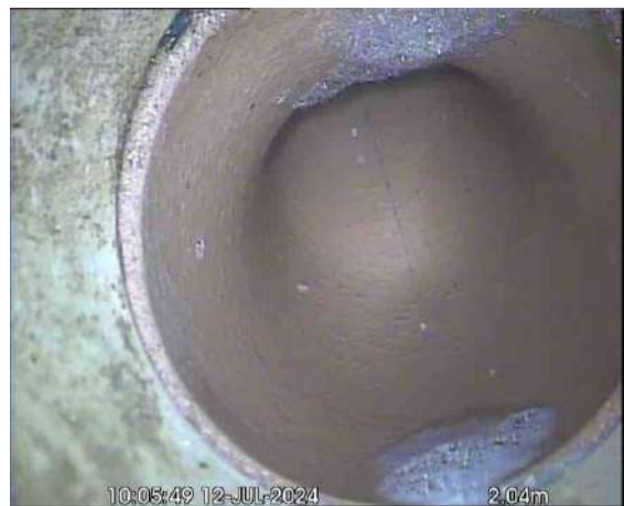
W_CX_96eda4f4-1bbb-49c3-bdf5-b6f3418d49e6_20240725_090429_528.jpg, 00:00:47, 2.04 m Line deviates up, REST BEND
