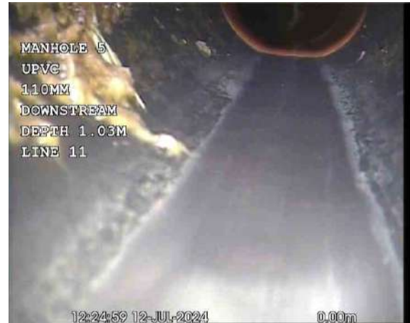
MH5X_04a04489-4146-4ad3-b2c5-d7ff96abe544_20240725_094519_970.jpg, 00:00:29, 0.00 m Water level, 0% of the vertical dimension
