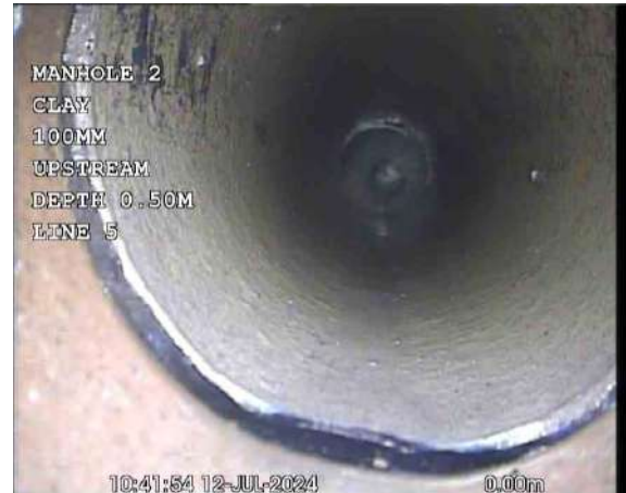
REDUNDANTX_e8cb558e-dafc-4f69-9ea3-26872ca7b2b2_20 240725_091117_148.jpg, 00:00:25, 0.00 m Water level, 0% of the vertical dimension
