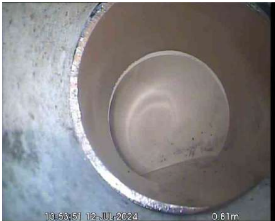
SVPX_6126ff3a-8feb-42cf-b4a8-289a35627abd_20240725_095243_344.jpg, 00:00:43, 0.81 m Joint displaced, medium
