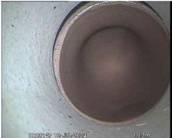
W_CX_1865770f-a7a0-438a-95c3-9da68d53db4d_20240725_090701_492.jpg, 00:00:39, 1.13 m Joint displaced, medium
