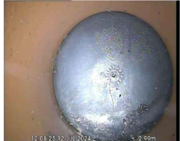
CAPPED OFFX_dc97001a-2078-4b93-b9a2-163b14f502db_20240725_093522_395.jpg, 00:01:03, 2.99 m Survey abandoned, S/A - CAPPED OFF
