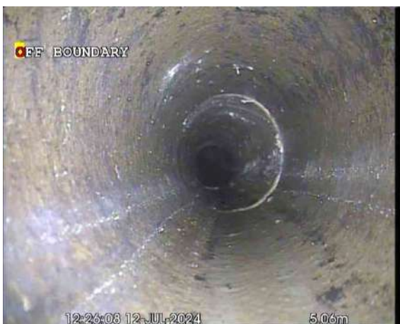
MH5X_7a719423-7b10-4cb5-9e10-35a6d7d11f95_20240725_094749_245.jpg, 00:01:36, 5.06 m General remark, **BOUNDARY POINT**
