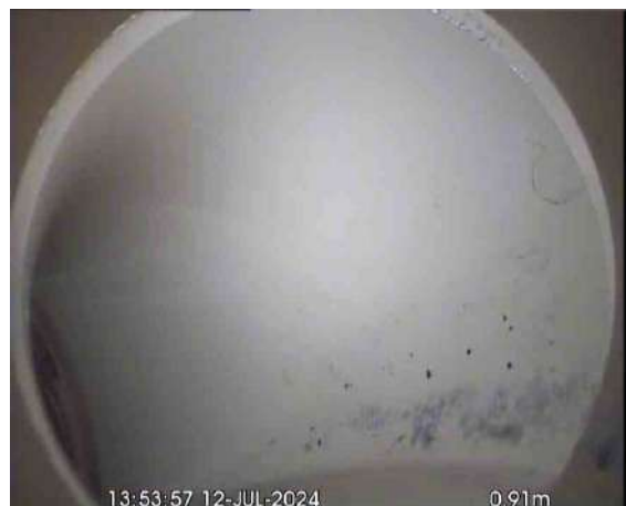
SVPX_1a7c91c5-7811-4395-aac0-3828833b4982_20240725_095342_984.jpg, 00:00:49, 0.91 m Line deviates left
