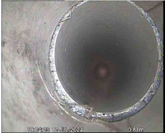
GULLYX_be408751-b267-4dcb-87b2-47920da53df0_20240725_090226_317.jpg, 00:01:01, 0.81 m Joint displaced, medium
