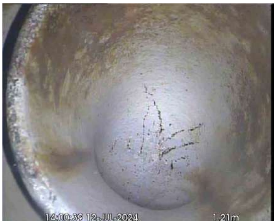
GULLYX_0146e961-7b26-494e-83c0-d047bf27c81e_20240725_101142_978.jpg, 00:00:31, 1.21 m Finish node, gully, reference: GULLY
