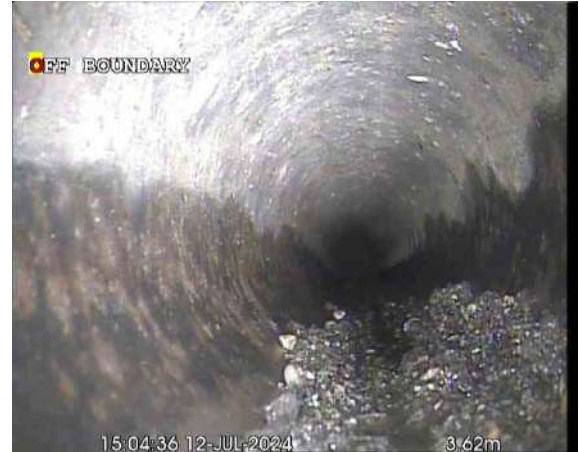
MANHOLEX_d574a494-dbda-46c8-9c0c-5e761cd3587d_2024 0725_102253_591.jpg, 00:01:02, 3.62 m General remark, **BOUNDARY POINT**
