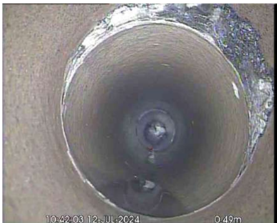
REDUNDANTX_0df9520d-4cc8-45ca-b8b9-6ea8c8cc1138_20 240725_091130_965.jpg, 00:00:34, 0.49 m Joint displaced, large
