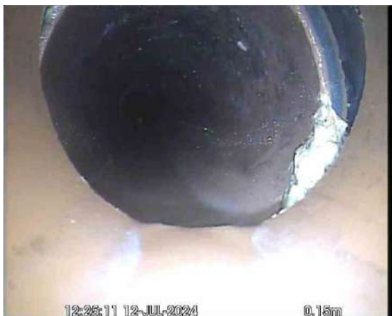
MH5X_a67b5490-9c73-459b-9229-8a05c12ea946_20240725_094558_658.jpg, 00:00:41, 0.15 m Joint displaced, large
