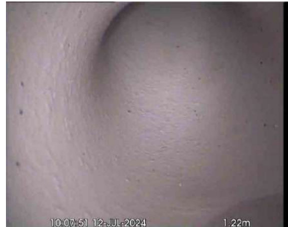
W_CX_e67dc308-cdad-4b4f-8f22-12bae3fd920a_20240725_090718_061.jpg, 00:00:43, 1.22 m Line deviates up, REST BEND
