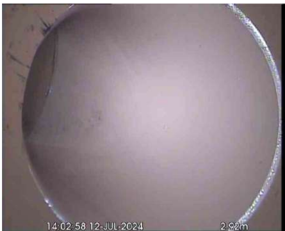
GULLYX_0fb9ef59-34cb-4c01-8650-9407a85952f5_20240725_101359_633.jpg, 00:01:09, 2.92 m Line deviates left
