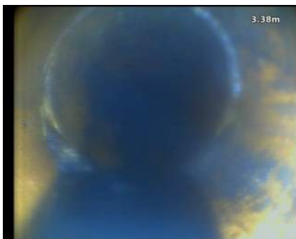
Observation [8]: DROPPED PIPE
