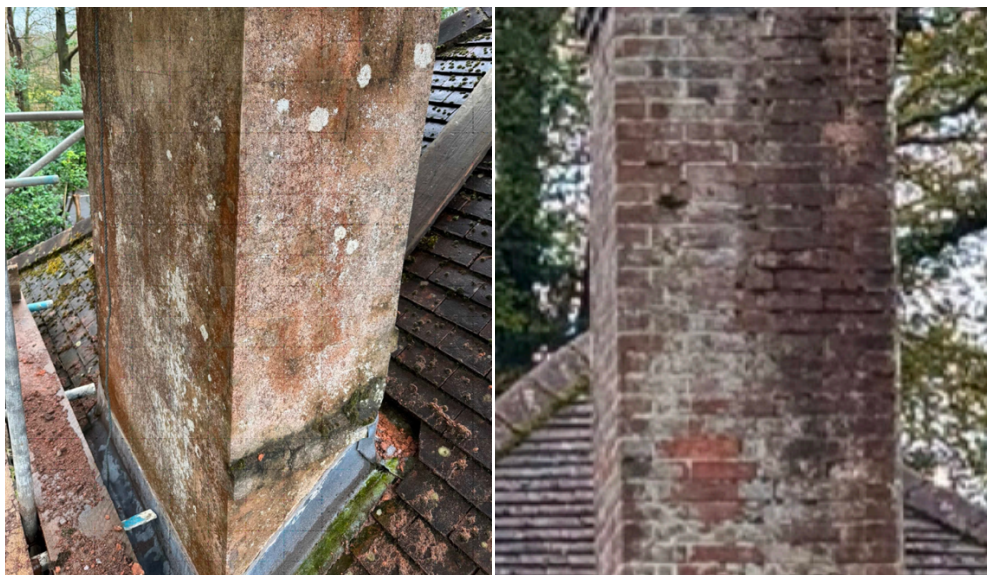
The south stack coated in render and the northern stack damp with salts.
