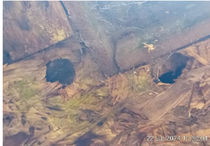
Figure 19: Example of gaps in chipboard covering eaves.
