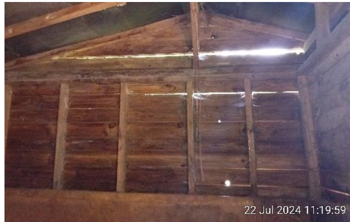
Figure 20: Example of gaps between timber planks.
