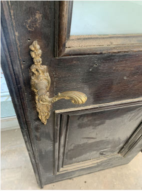
Image of existing non original Ironmongery. Ironmongery from Doyle era alterations.
