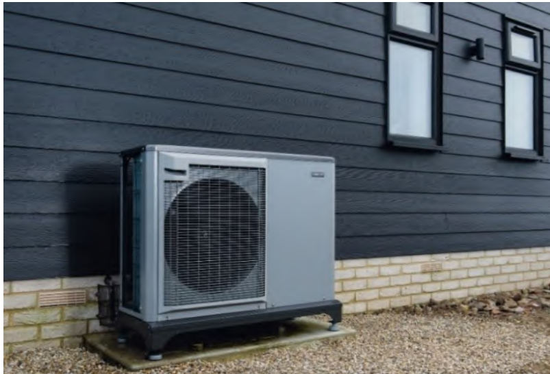
Figure 5.1: ASHP – External Unit
