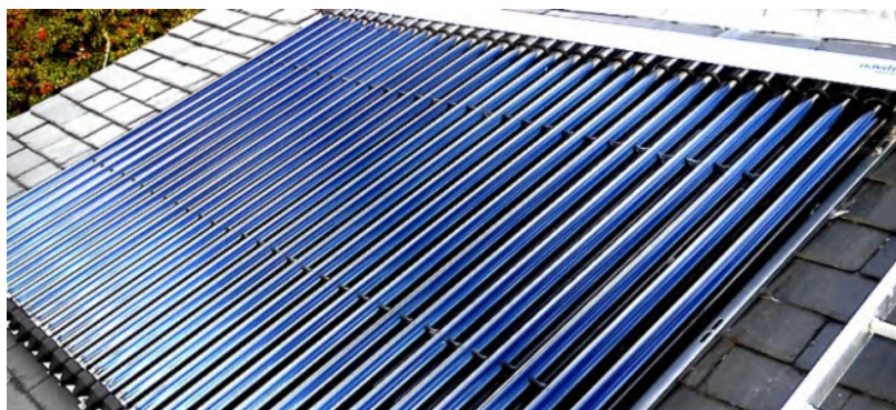
Figure 5.5: Evacuated Tube Solar Thermal Panels
