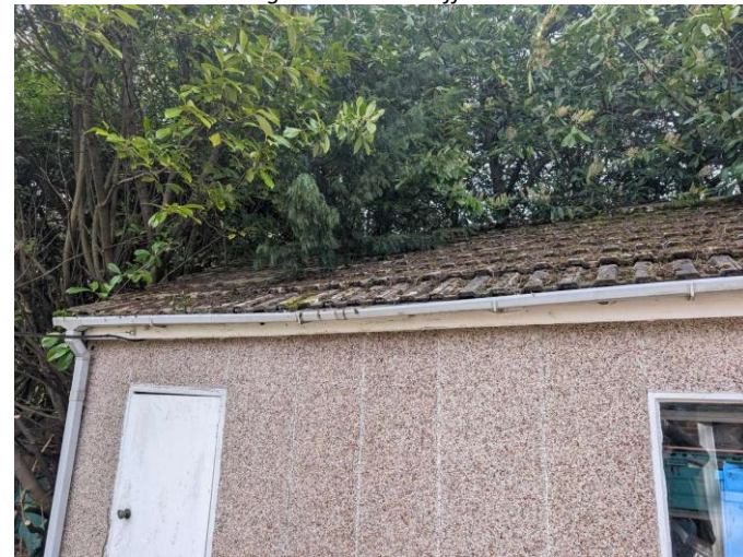
B2 tightly fitted roof tiles.
