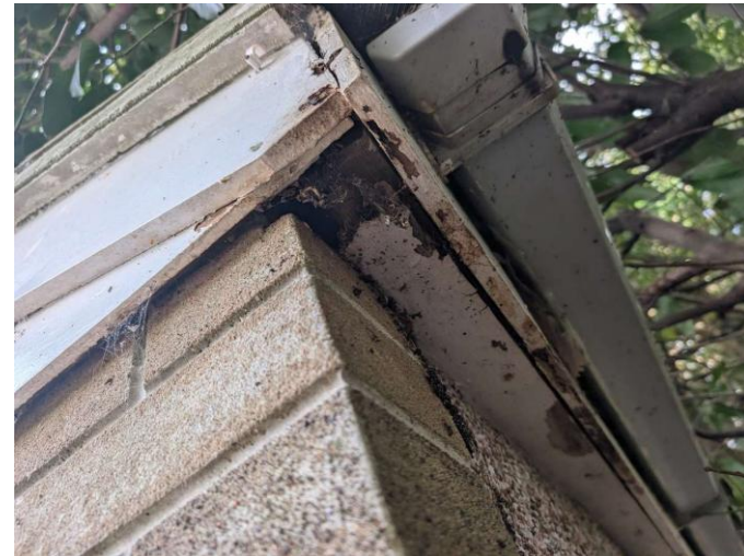
B2 aged but intact soffit boxes
