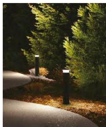
● Black bollard lighting doubling up as EV charging where required
