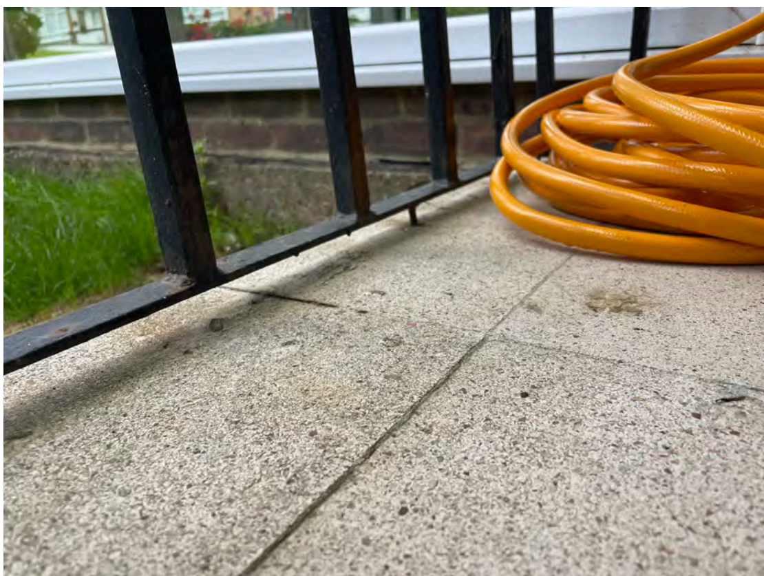
28 - No. 8 Byron Court Balcony gap and screw fixing at base of handrail
