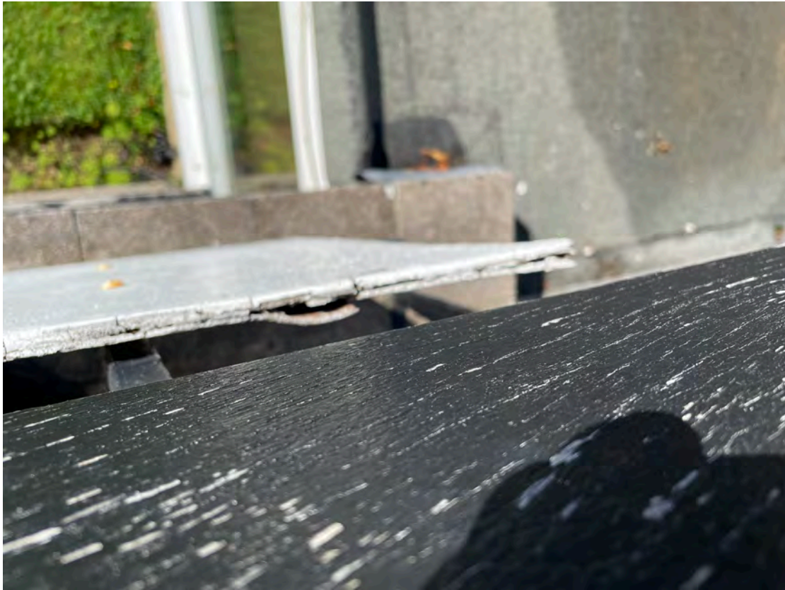
19 - No. 10 Chaucer Court Balcony delamination of infill plyboard panel
