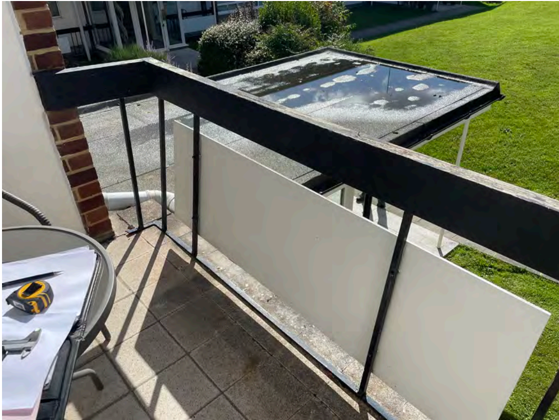
11 - No. 9 Chaucer Court Balcony east side with extra post to the front corner
