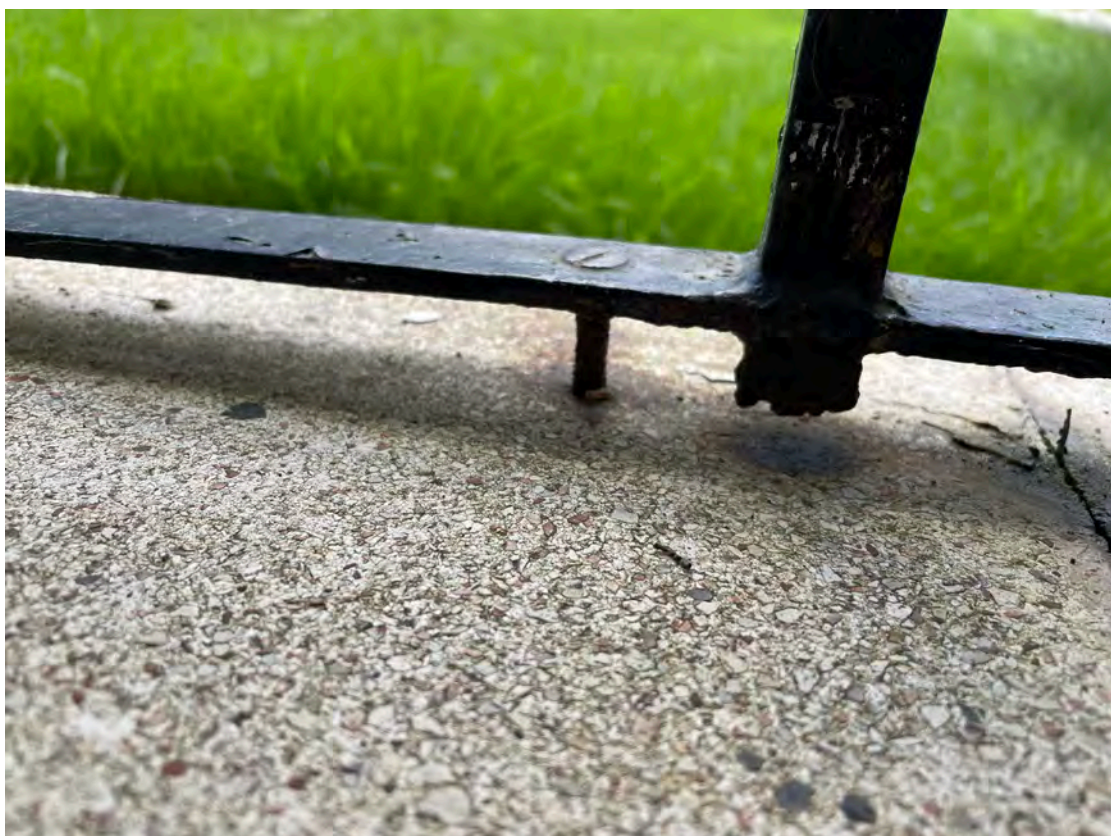
29 - No. 8 Byron Court Balcony gap and screw fixing at base of handrail
