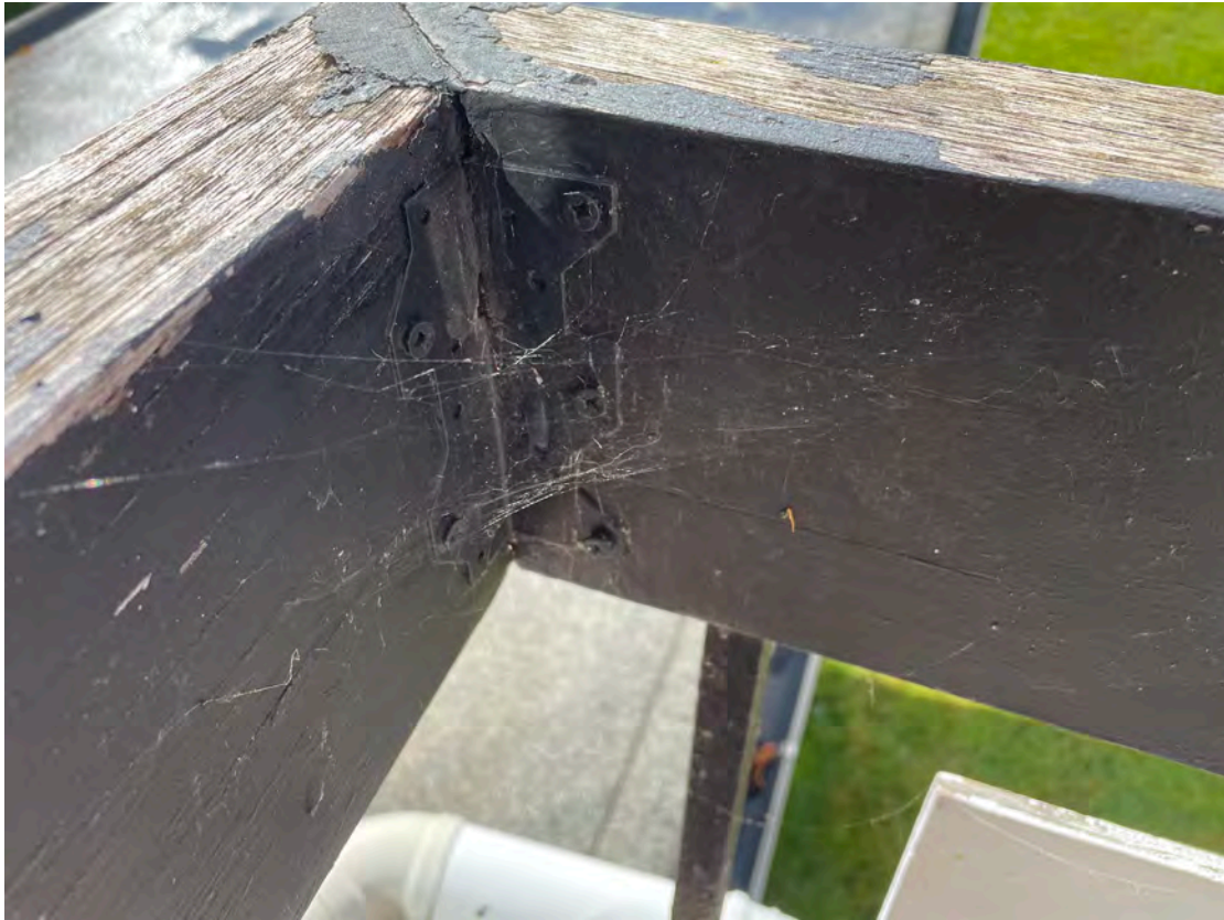
13 - No. 9 Chaucer Court Balcony east side corner handrail bracket
