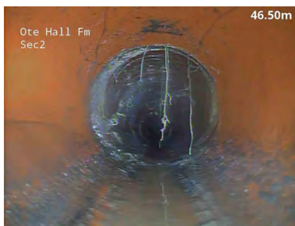
16, 00:02:21, 46.70 m Roots, fine at joint
