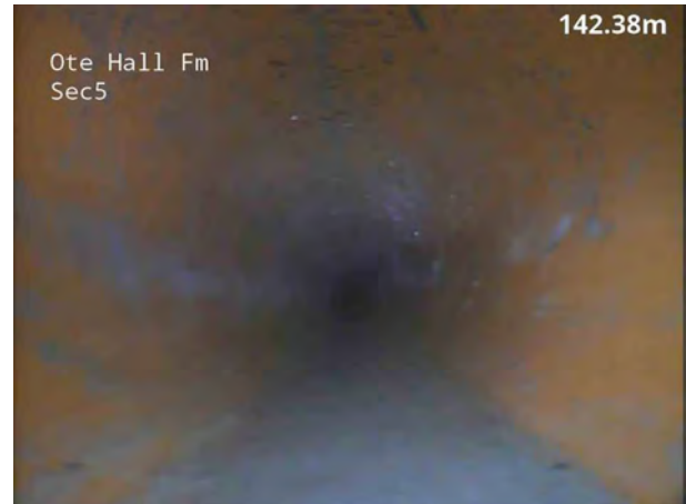
2, 00:05:11, 142.40 m Survey abandoned, Unable to reach chamber, to come up from FW2
