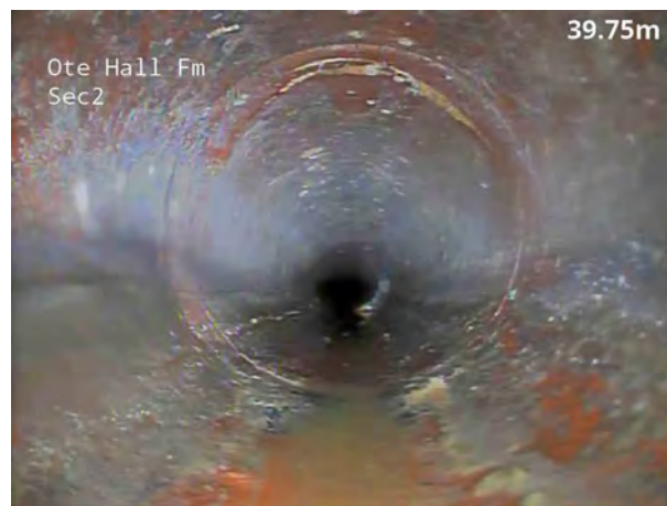
12, 00:03:18, 39.90 m Fracture, circumferential at joint from 12 o'clock to 12 o'clock
