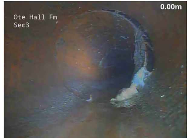
2, 00:00:11, 0.30 m Roots, fine at joint
