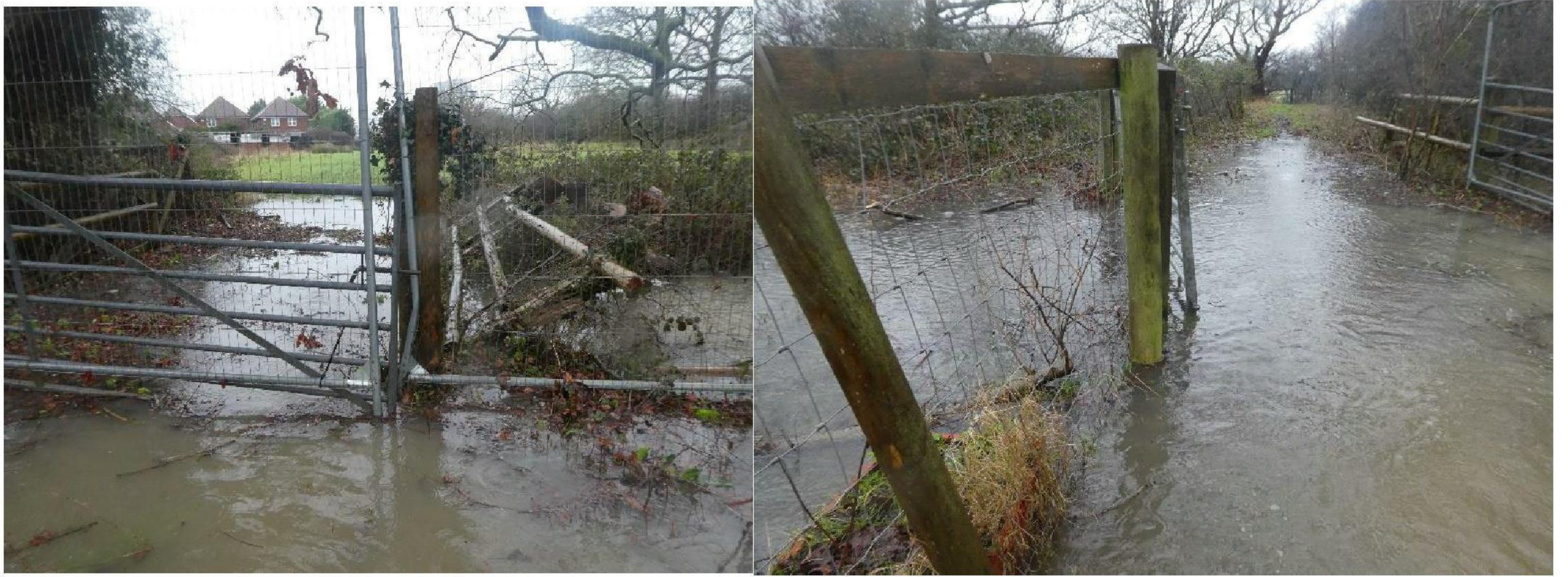
B- Flooded footpath by the bridge to the northern part of the site.27/01/2026 11:20am (Please note that this flooding is over 20cm deep in places and it is therefore not possible to distinguish which parts are actually the bridge, footpath or stream.)
