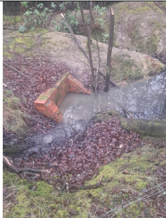
32. View of headwall and culvert along tributary watercourse flowing from northeast to southwest along
