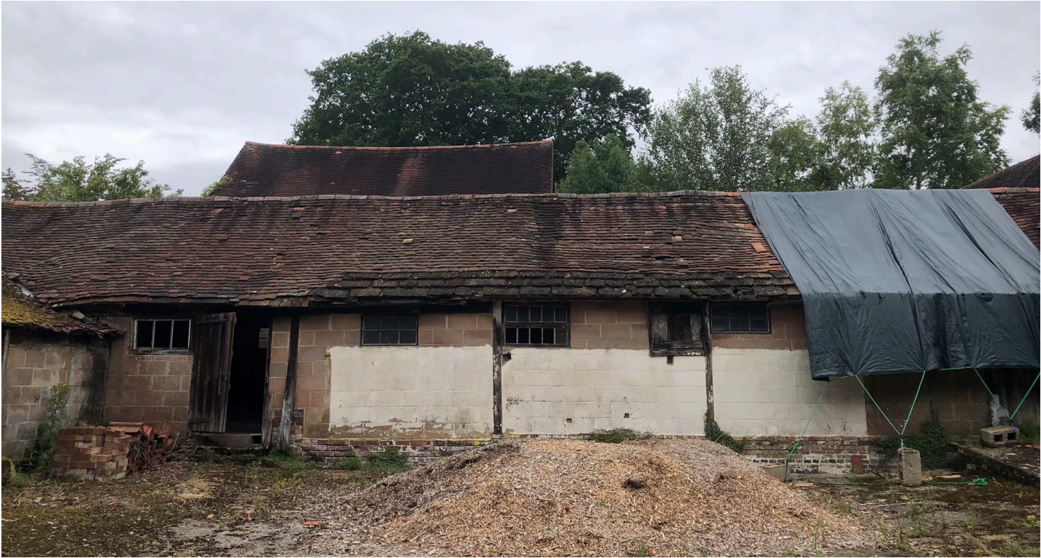
Cowshed, with existing roof in pressing need of repair and renovation
