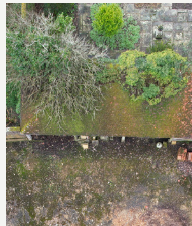
MOSS AND PLANTS OVERGROWN ON ROOF
