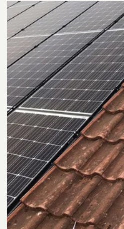
SOLAR PANELS THE STABLES
