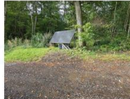
View 2. Solar panels located northwest of the south pod.
