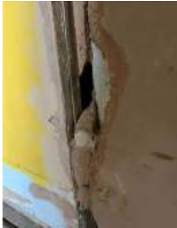
Poor quality bathroom wall before demolition
