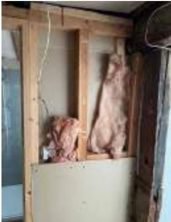
Poor quality bathroom wall build up exposed before demolition
