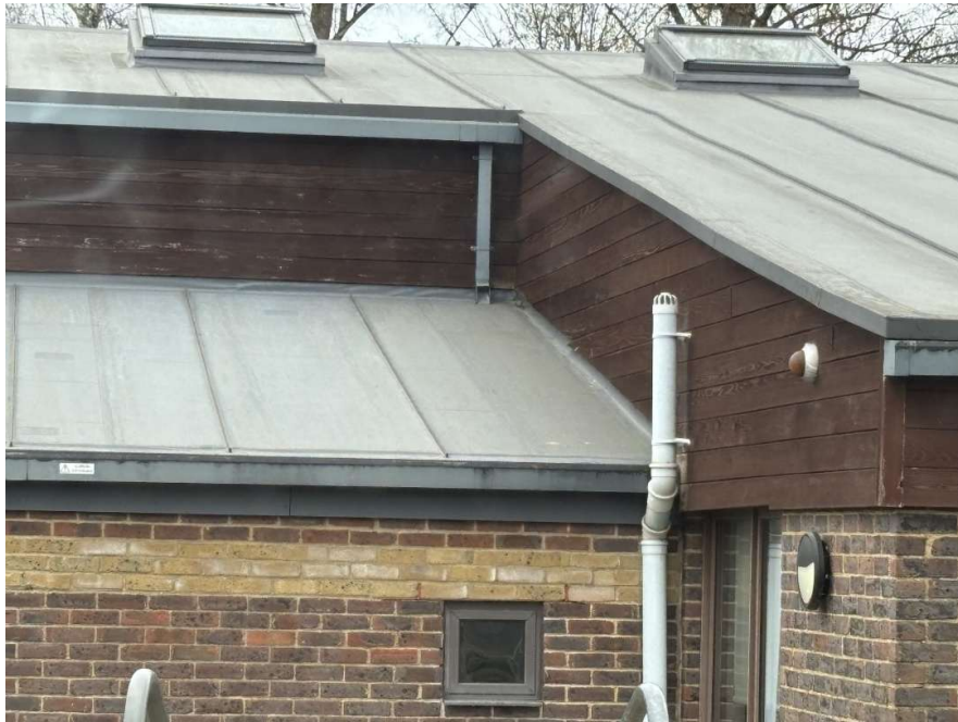
Figure 20 – Trinity Road, Hurstpierpoint Village Centre (significant cladding)
