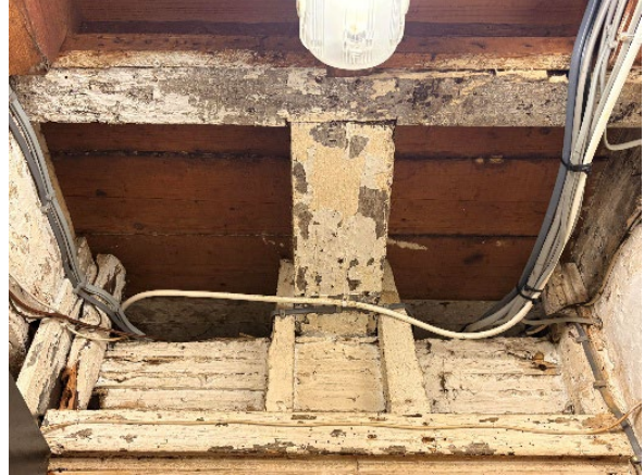
Figure 23: Gap above cellar door where fire stopping is to be carried out
