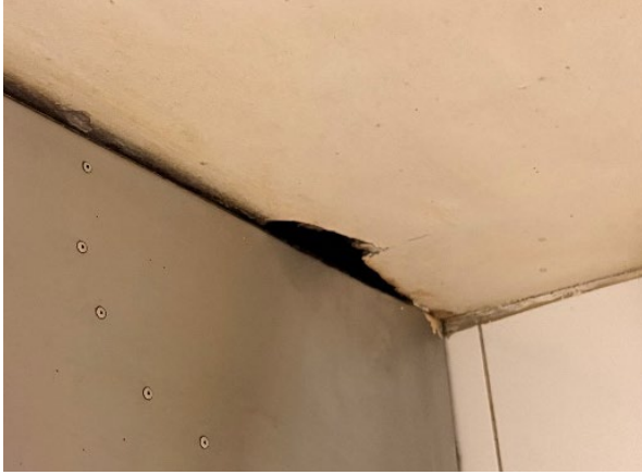
Figure 22: Gap above cellar door where fire stopping is to be carried out
