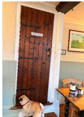
Figure 19: FD2 – The non-historic fire door with decorative cladding to be replaced
