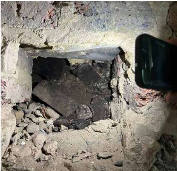
Ground floor living chimney breast assessment, opening from hall side. Chimney breast blocked up and not usable.
