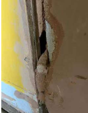
Poor quality bathroom wall before demolition
