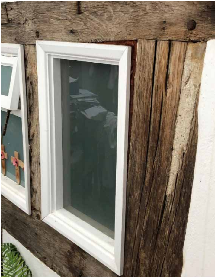
Pre-construction photograph of low quality casement window, west facade (ground floor). Foam around the frame visible.
