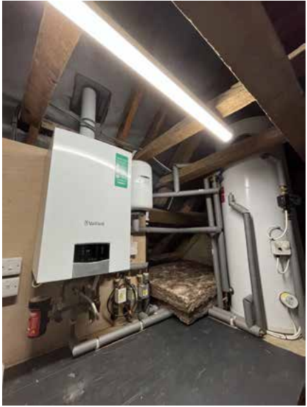
Recent photograph capturing the new water tank and boiler installed in attic
