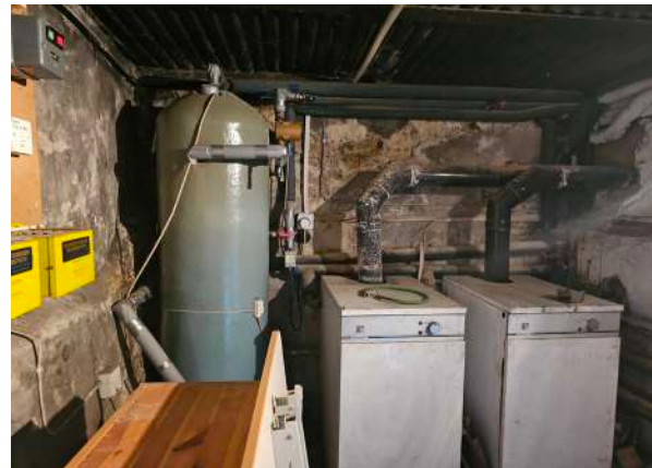
boilers to be replaced
