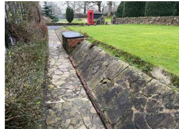
bin store and raked retaining wall to west to be rebuilt
