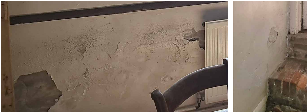
Lower walls with spalling synthetic paint and cracked cement render
