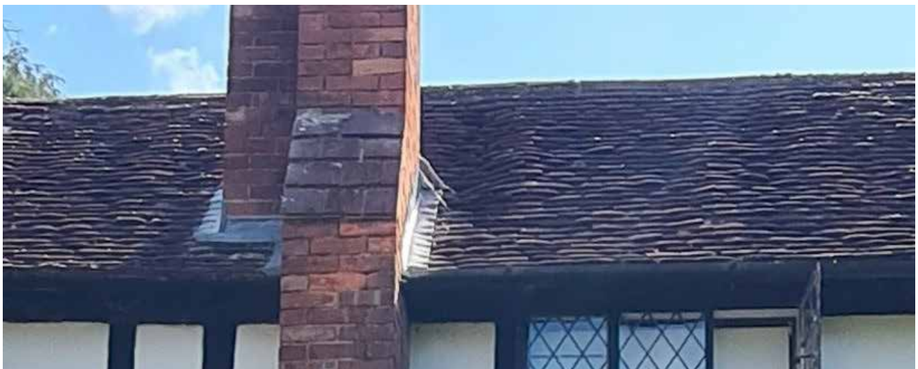
Sagging roof beside the south chimney stack and eroded pointing on stack's brickwork
