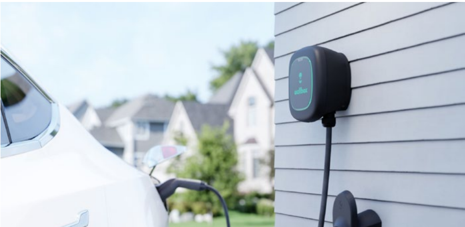
Electric Vehicle Charging Point
