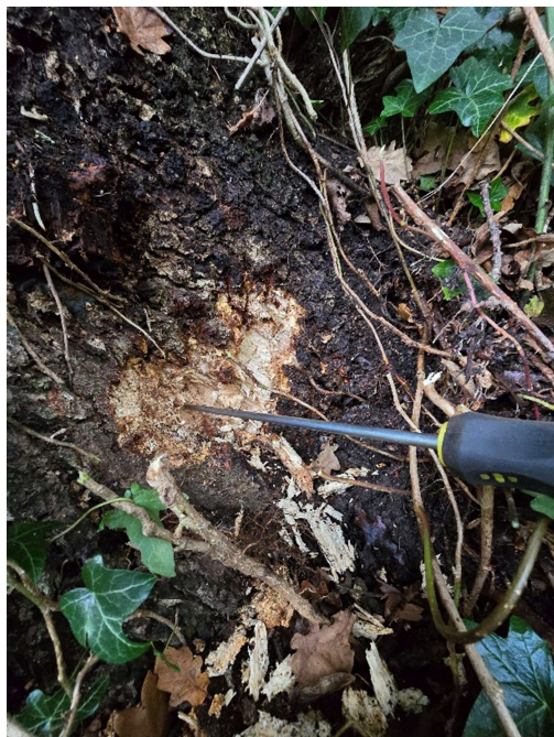
Photo B3 – Decay Probe Behind Bracket
