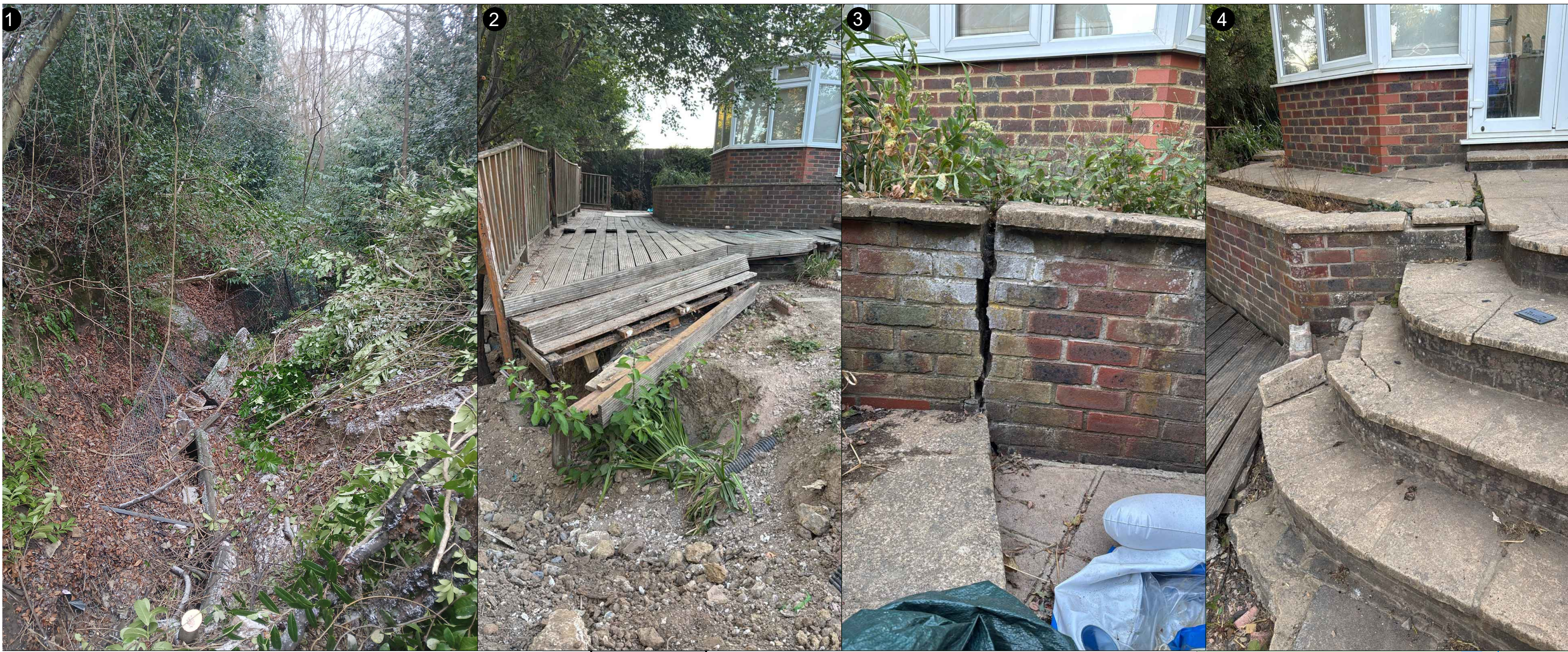
Images of Collapsed retaining wall and its effects on No.1 Alders View
