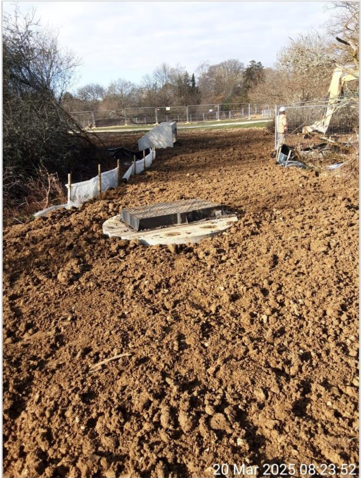
Photo 12 – Manhole S44 Hydro-brake
