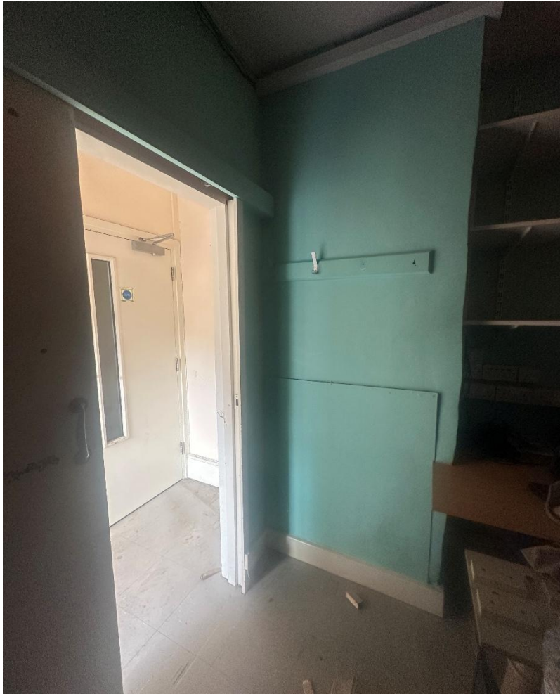
Image 1 – shows a picture of the stud wall from inside the storage cupboard and you can see that it has been built up abutting the chimney breast leaving a small unlit and unsympathetic space.
