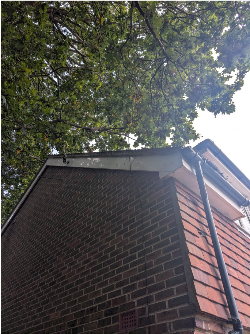
E1 Garage roof apex and overhead cable
