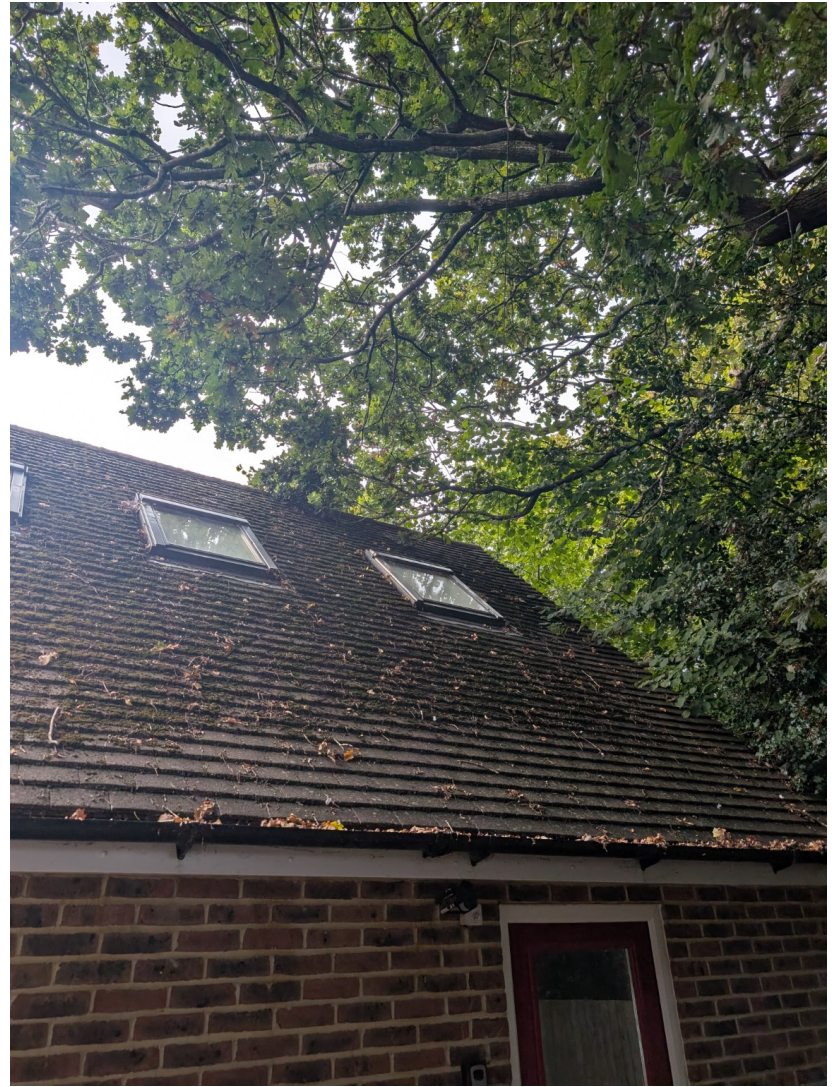
E2 Lower branches above pitched roof
