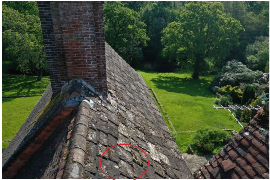
evidence of laminated and cracked tiles
