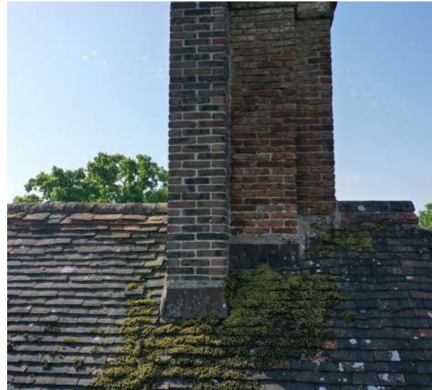
clay peg tiles, tile and half to verges and mortar bedded abutments. Note moss and lichen growth and areas of consequent spalling
