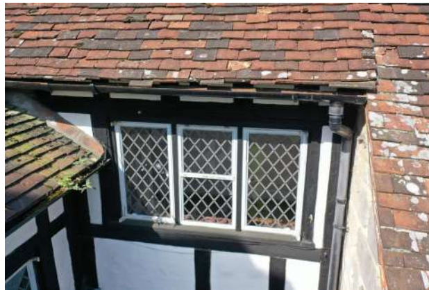
slipped tiles to the eaves
