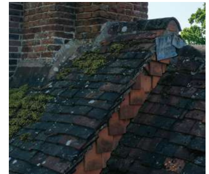
double lap tiles evident at verge
