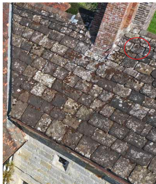
evidence of soakers in contrasting material
