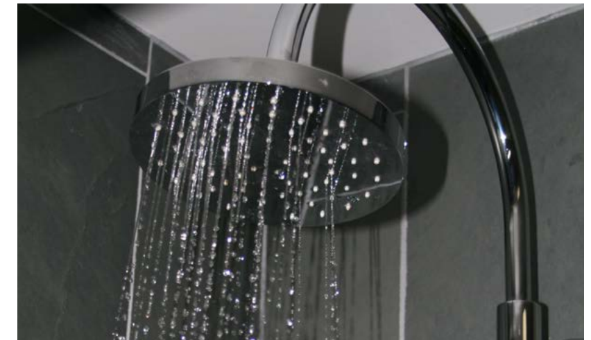
Low water usage fittings installed in all dwellings
