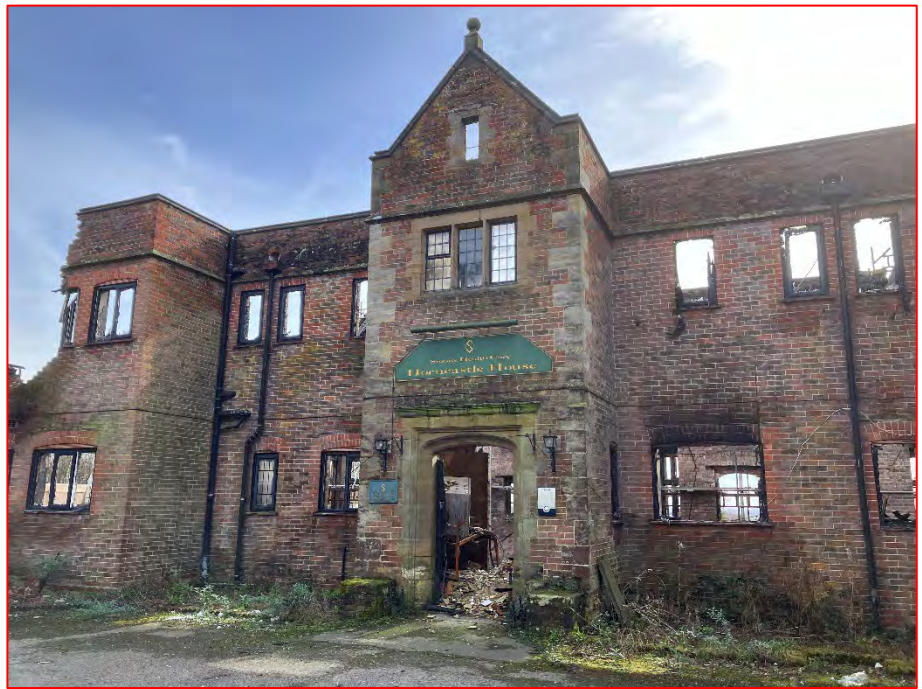
Plate 4 North elevation of fire damaged Horncastle House prior to demolition.
