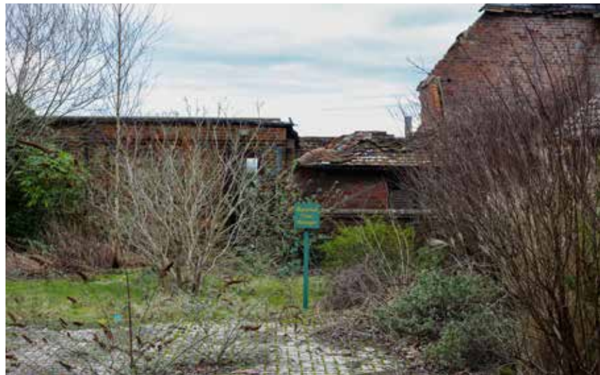
Image E: The planting around the staff car park is overgrown
