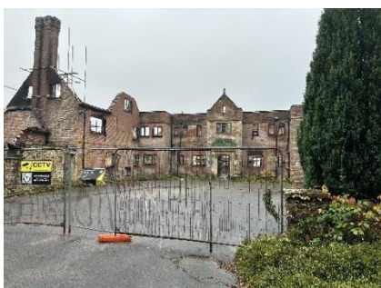
Figure 4: Front of main house following fire damage (prior to demolition)
