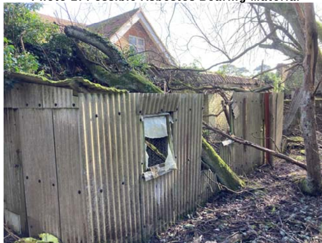
Photo 2: Possible Asbestos Bearing Material
