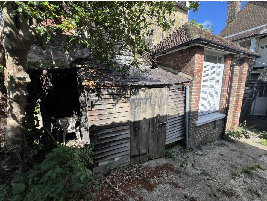
PHOTOGRAPH OF DILAPIDATED TIMBER-CLAD OUTBUILDING
