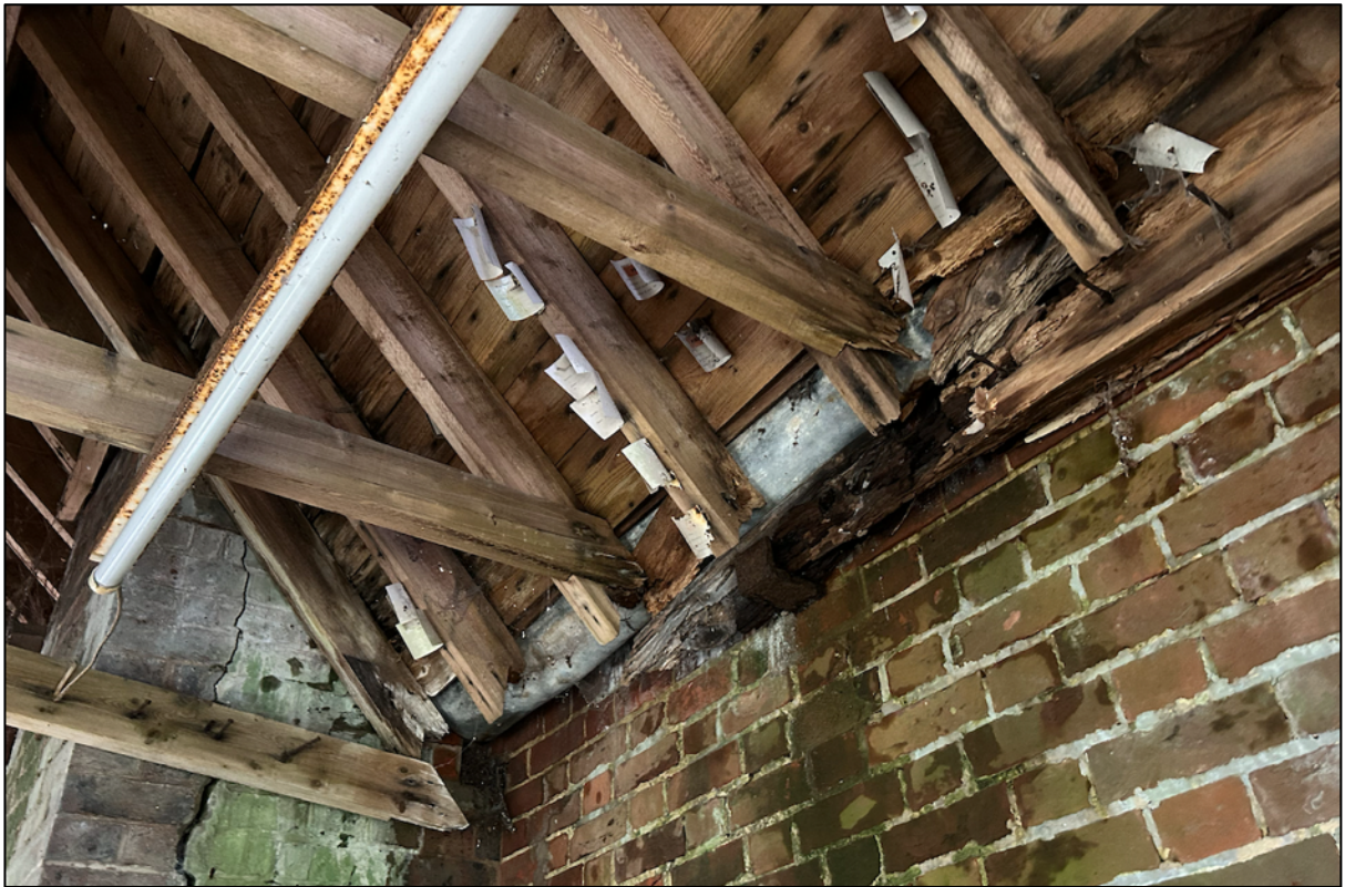
Photograph 5. A degraded section of roof on the western side of the building where the rafters have detached from the wall plate.
